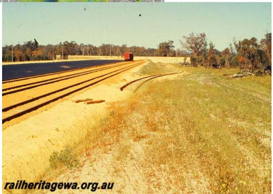
P09880 Bibra Lake, new yard, hard stand for interchange, standard gauge in background, remains of Jandakot branch at side of yard. FA line.
